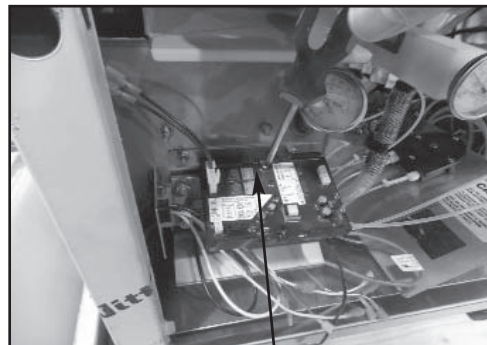
Replacing the ELAN thermostat.
